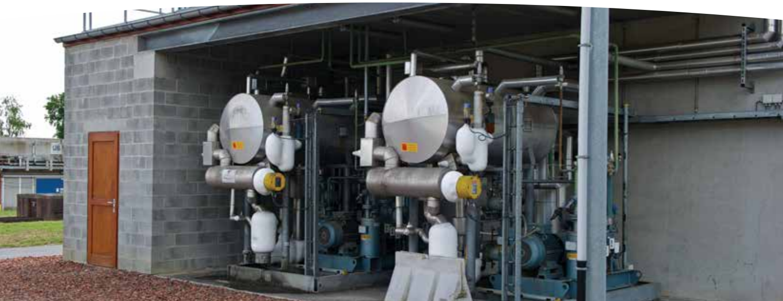
Two cooling units, alternately operating, fully independent of each other
